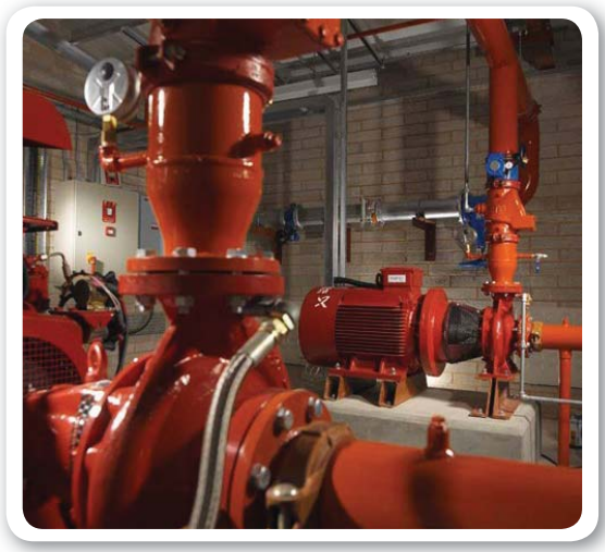
Fire Water Pumps and Tanks
